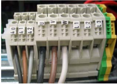
Fig. 21: Power supply terminal board
